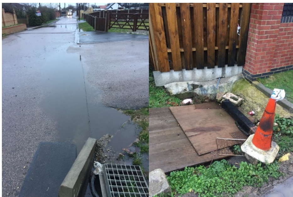
Figure 3-19: Surface water and foul drainage issues – Hovefields Avenue
