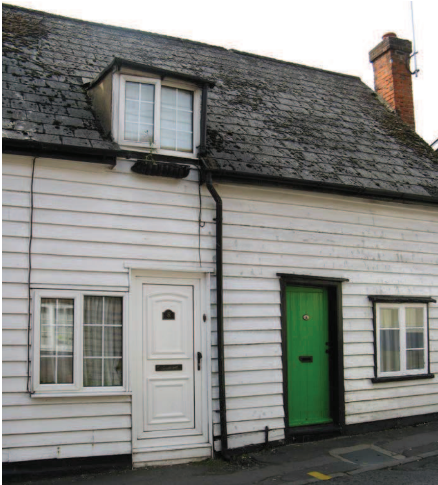
This 14th Century Grade II* Listed Building has been seriously compromised by inappropriate UPVC double glazing and enforcement action can be sought.
